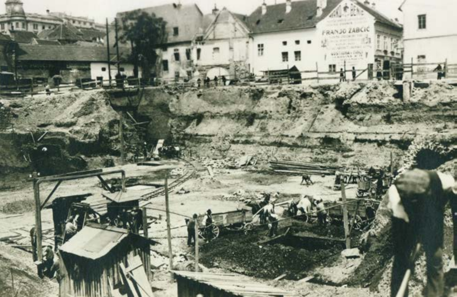
Building the foundations for the new Dolac Market, Zagreb, V. Horvat, UZKB – F, the Ministry of Culture
